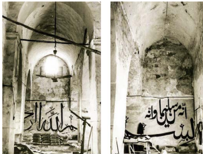
Picture 6. Hand-drawn calligraphy in the Harim during the repair of foundations in 1956 (Archive of the General Directorate of Foundations)
